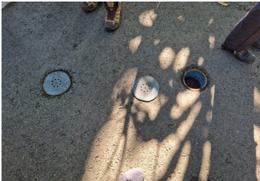
Soil compaction study methods digging holes and perforated PVC pipes in road pavement
